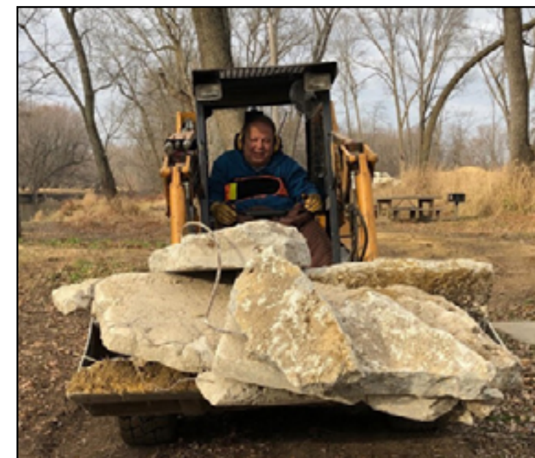
Roger Schamberger tests the metal of his skid loader as he places erosion protection at a Pecatonica River fishing pier. All photos: Joe Ginger
