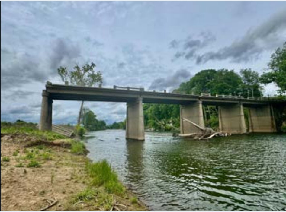
Damaged Bridge: Corby Bridge on the Nolichucky River, severely damaged by Hurricane Helene, is slated for replacement and will include new river access. Photo: Jeffrey Duncan
