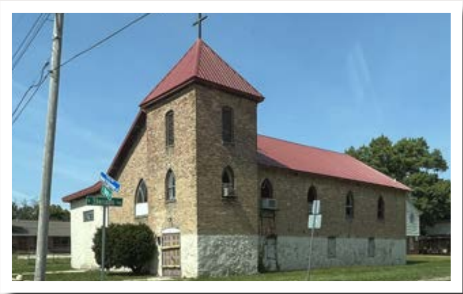
St. Paul Missionary Baptist Church, original building with replaced roof: The church was permanently closed and boarded up due to flooding. Photo: Cheyenne Morgan
